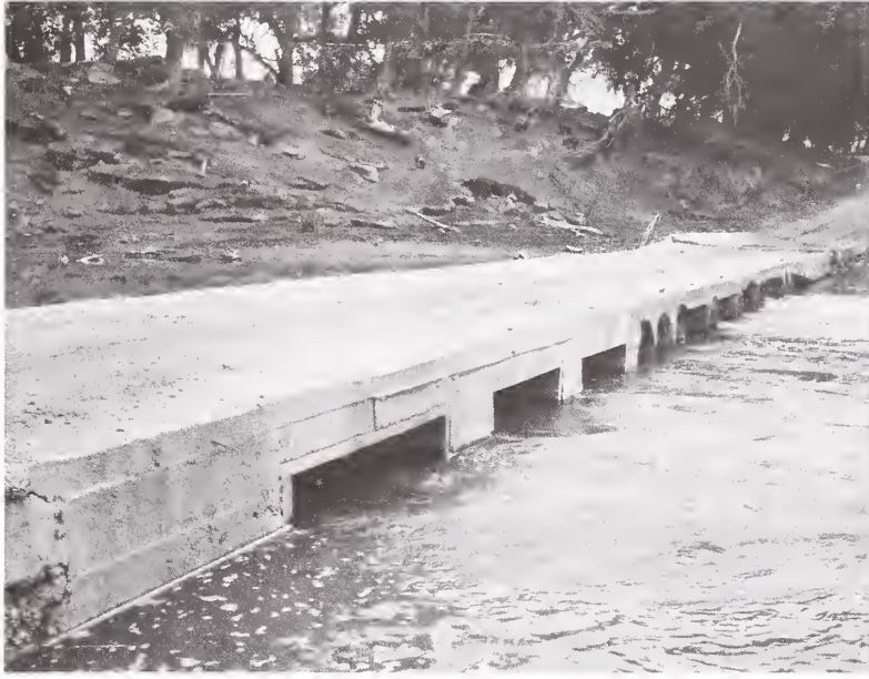
The Milk River Ford Box Culvert is one earliest remaining structures of this type in Montana. It is typical of pre-Commission box culvert design (Illustration by John Robinson).
